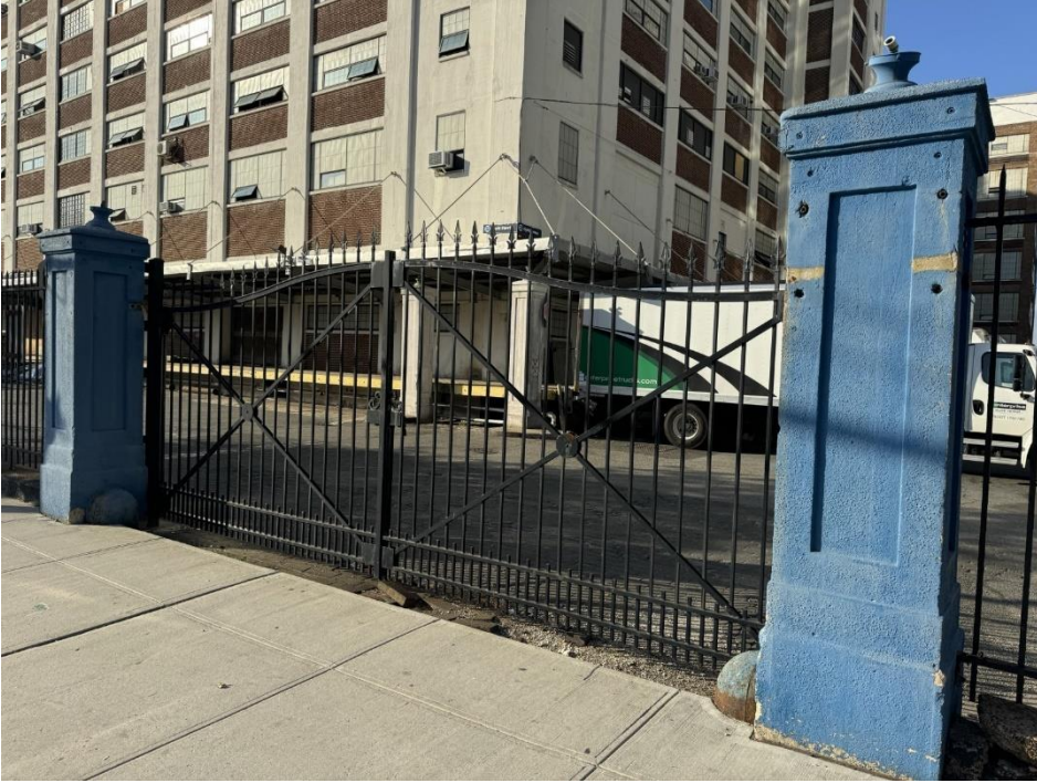
First historic gate between two blue columns: 24.5' W x 100" H. Section A6
