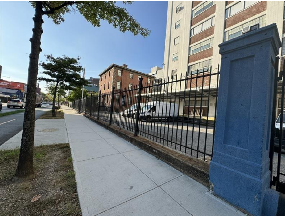
Long section with Building 92 (red brick) in the distance: 99.5' W x 82" H. Sections C35-38; C36-41 not pictured)
